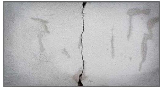
Fig. 4. (a) Medium crack (1-2mm) (constrofacilitator.com)
