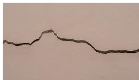
Fig. 5. Wide crack (>2mm) (loveproperty.com)
