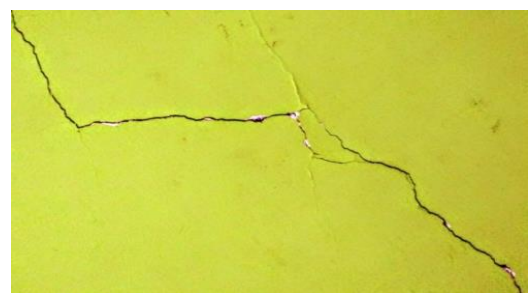
Fig. 4. (b) Medium crack (1-2mm)
