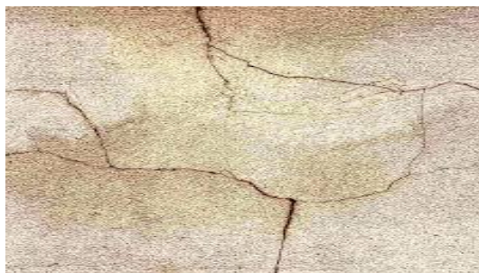
Fig. 3. (a) Thin crack (<1mm) (gharpedia.com)
