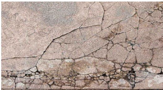
Fig. 2. Non-Structural cracks (gharpedia.com)
