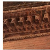
Lions Head Exposed on Cornice
