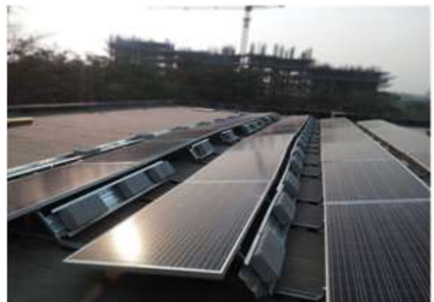
Figure 2: Solar PV Plant on rooftop of NCB-H
