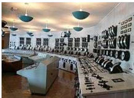
Figure 2 a Pre-DCS/SCADA Era Central Control Room
