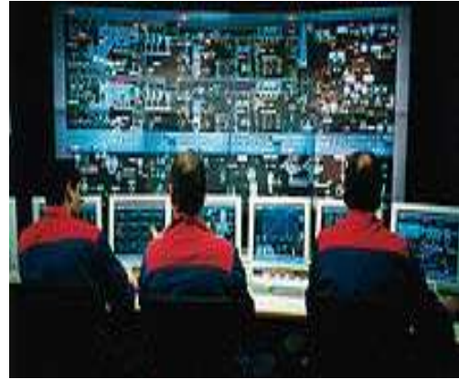
Figure 3 a DCS Control Room
