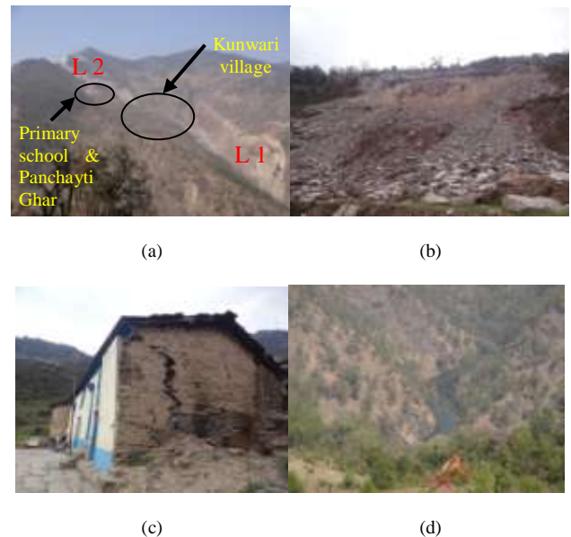
Fig. 2. (a) Kunwari village between landsliding zones (b) rock slide (L2) upslope of village (c) wide cracks in the house wall indicating active slope movement (d) lake formation on Baura Gad below Kunwari village due to landslide
