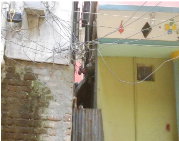
Fig. 2. Risky wire and No side spacing (Picture has taken from Farmgate)
