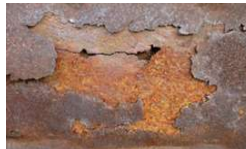
Fig. 4. Corrosion effect in boiler[16]
