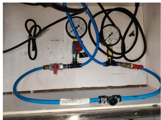
Fig. 9 Pneumatic network and pressure gauge
