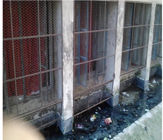
Fig. 12. Plumbing hazards in Mirpur
